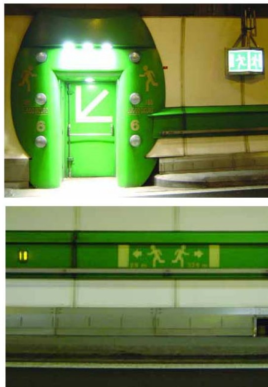
Figure 1-12 Emergency Exit (FHWA, 2006)
