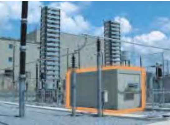
Fig. 5.4.3-1: Active DC filter on site (Tian Guang HVDC project)
