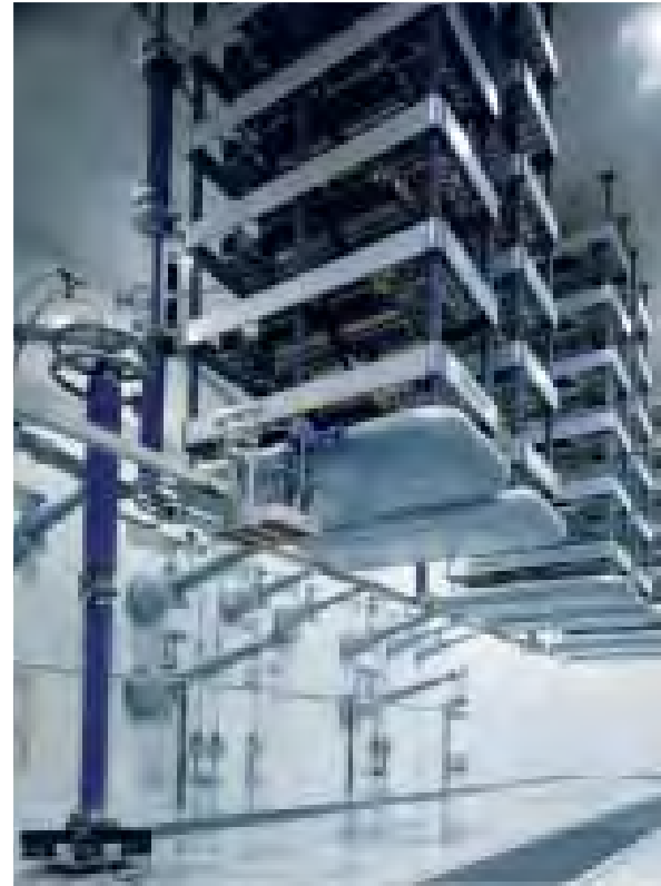
Fig. 5.1-8: Converter valves Sylmar HVDC station, Los Angeles, USA
