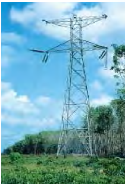
Fig. 5.6.1-1: DC transmission line (bipolar tower 300-kV link)
