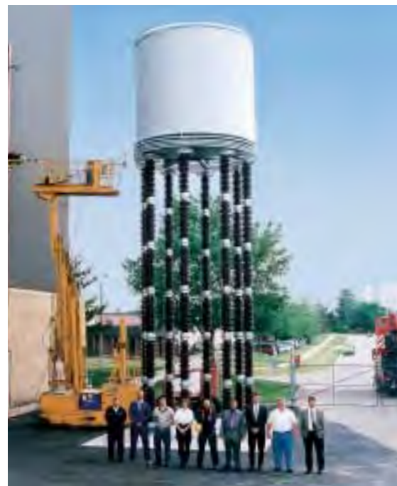
Fig. 5.3-2: Air-insulated smoothing reactor – Tian Guang project
