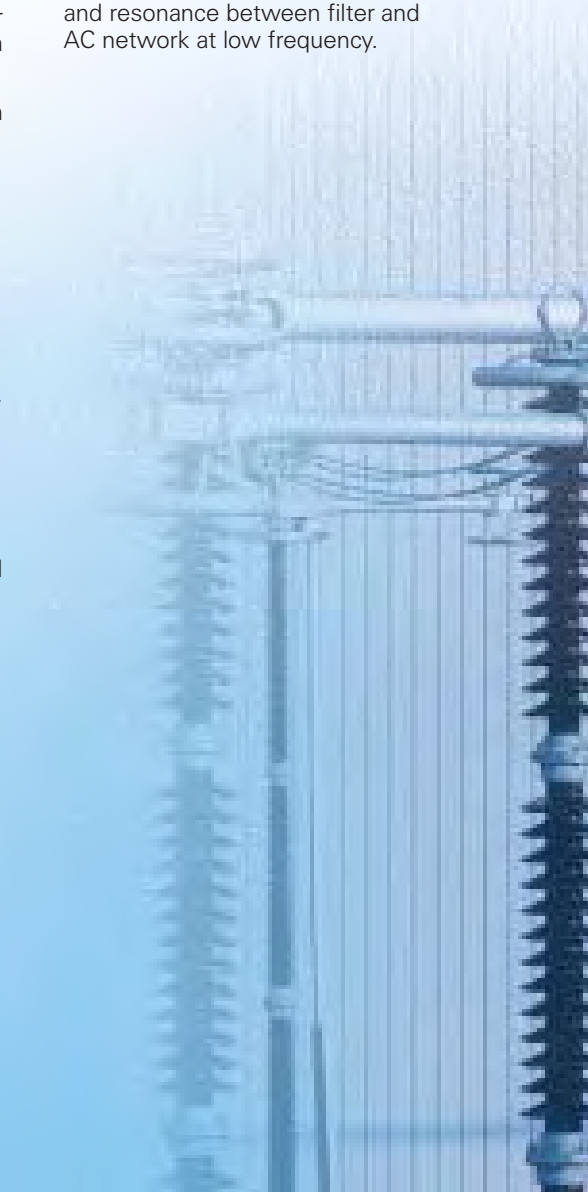
Fig. 5.4.2-1 DC filter of Guangzhou/China
